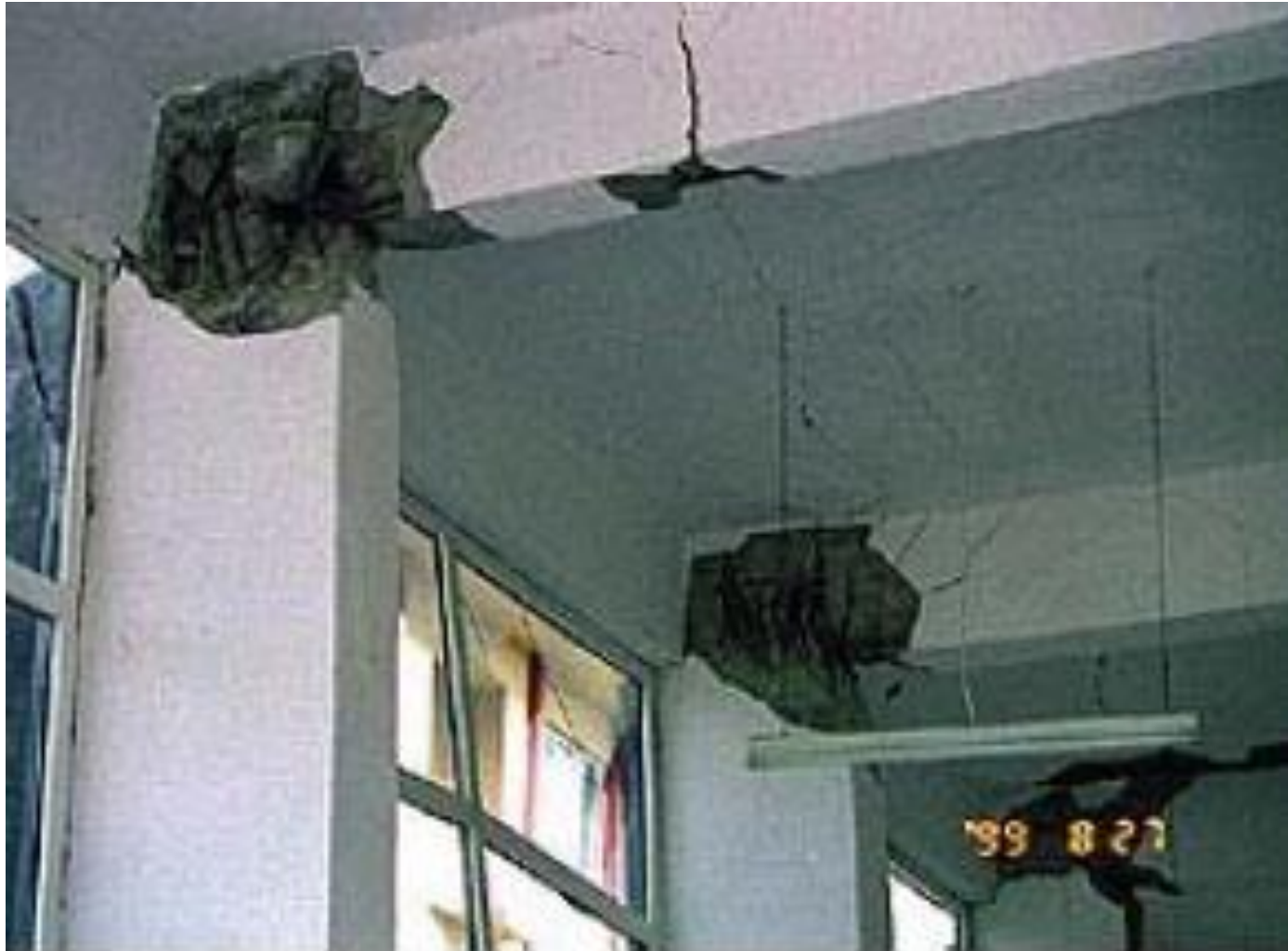
Figure 3-36 Damage to a new moment-frame beam-column joint
