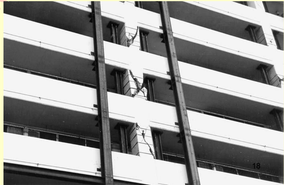
Reinforced-concrete columns severely damaged in the Northridge earthquake, Champagne Towers, Santa Monica, CA.
