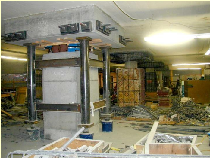
Column jacking and stressing hardware
