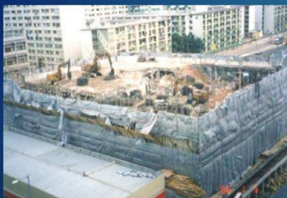
Typical sectioning/ sequencing arrangement of work during demolition – demolish from one side to the other side of building
